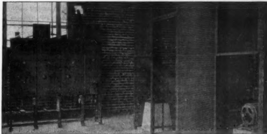
FIG. 9—VIEW OF ELECTRIC CONTROL BOARD SHOWING WOVEN WIRE PARTITION BETWEEN MOTORS AND RECTIFIERS AND TRANSFORMERS
